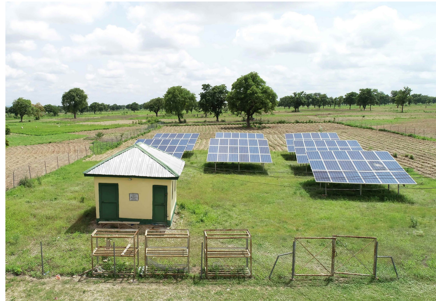
A 24kw mini-grid PV solar farm project in Bisanti Village, Niger State, Nigeria installed by Green Village Electricity (GVE). GVE provides 7,400 households in thirteen rural communities with reliable access to electricity.
